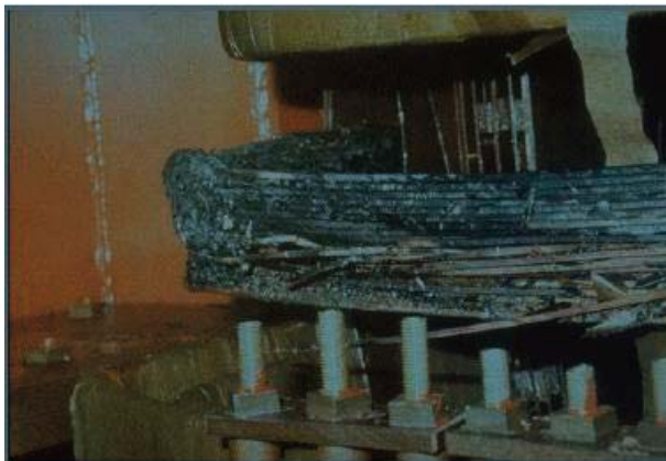
Figure 7 Picture of a transformer damaged by overheating
